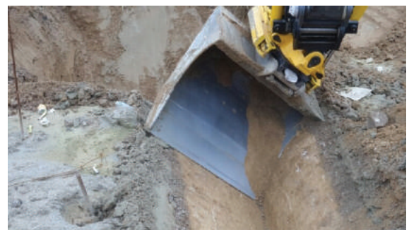
Electrical cord and puddle
